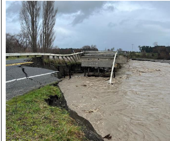
26 June 2023: SH50 at Waipawa bridge
