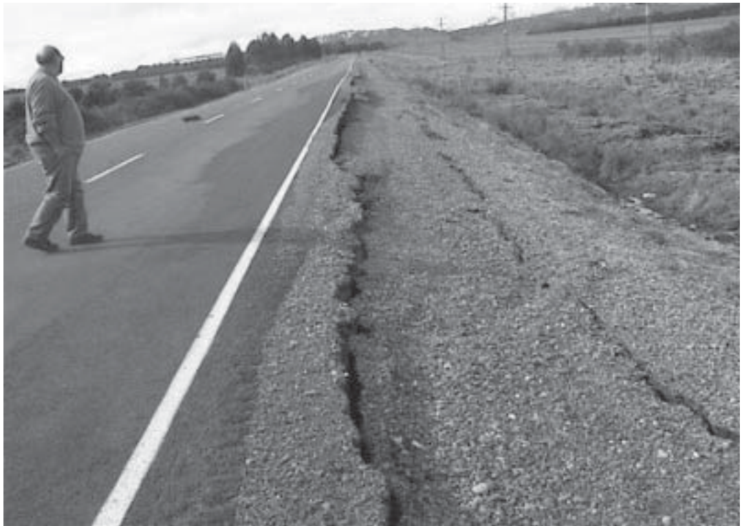
Southland District Council engineer John Cook inspects slumping on Hillside Road near Manapouri, caused by the earthquake.
