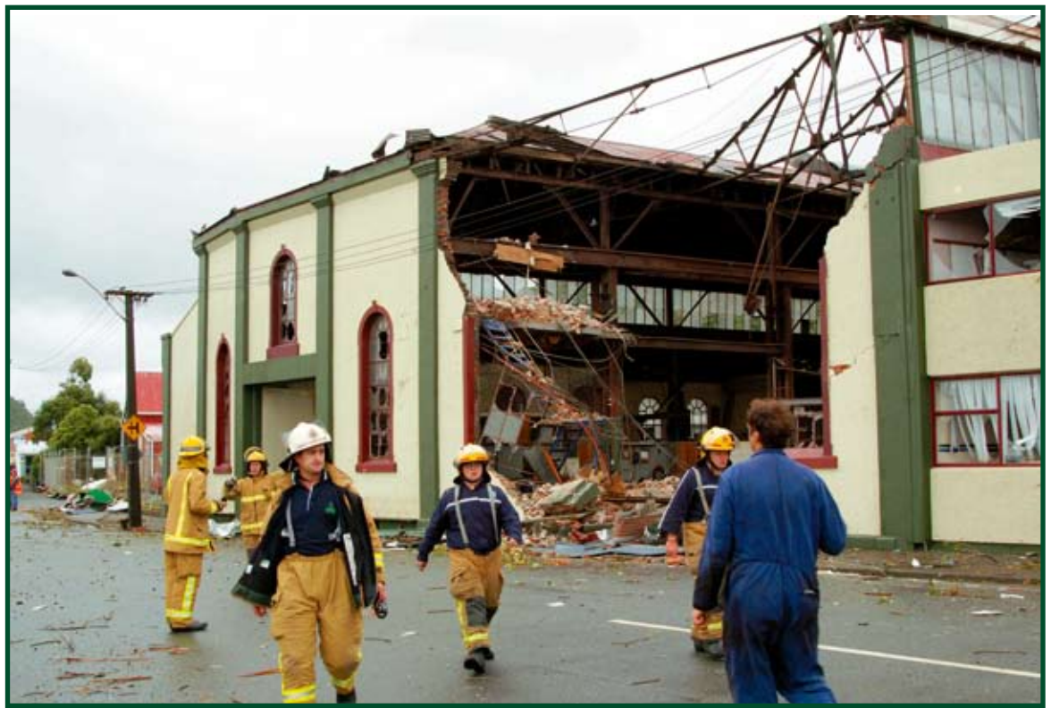
Severe damage after a tornado swept through Greymouth in March. Picture by the Greymouth Evening Star.
