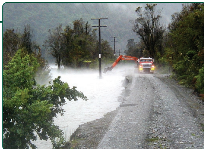
Erosion of the floodbank on the south side of the Waiho River just downstream of the holiday park area.
