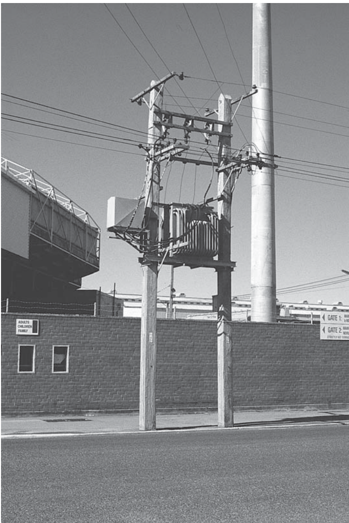
Typical Pole Mounted Transformer - Civil Defence
