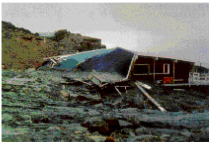
The Staircase Kiosk at Whakapapa ski field was structurally damaged by the June 1969 lahar and was later removed. Note how the rear wall was shoved in, part of the roof collapsed and later portions of the lahar washed up onto the fallen roof. Photo by V.E. Neall
