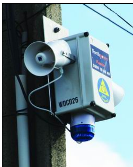
Figure 31: Example of a siren installed in Northland. Image from the Northland Regional Council website [46].
