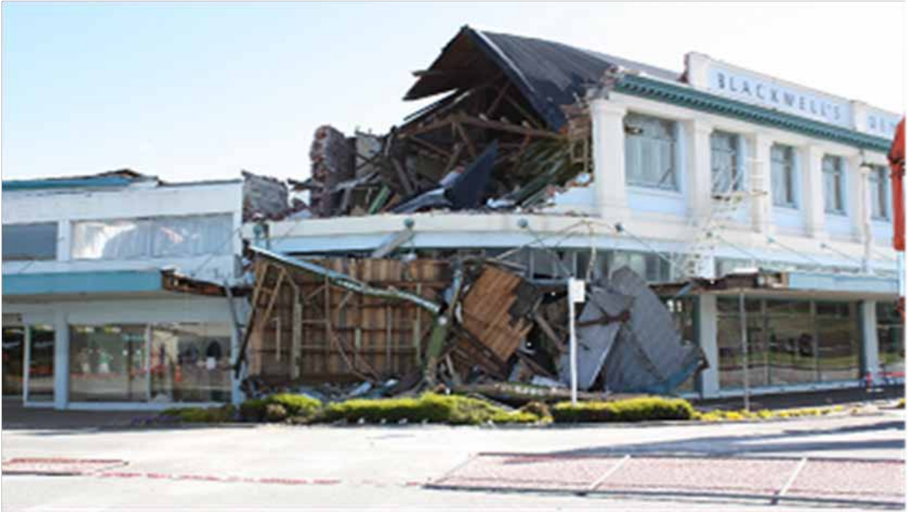
Blackwell's iconic department store in Kaiapoi after the 2010 earthquake. Rebuilt quickly to boost community morale.
